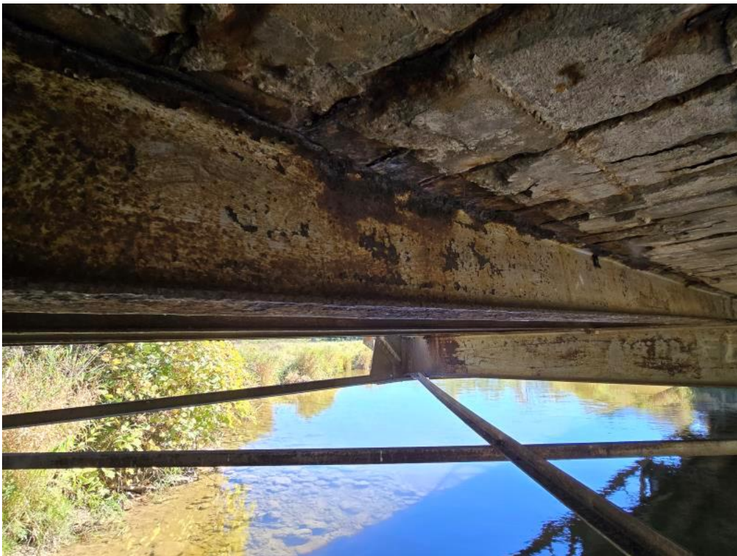
North Bay Stringer Corroded Top Flange
