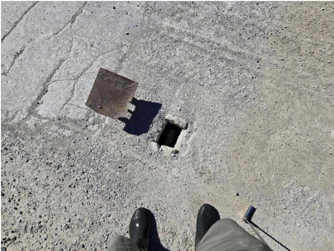
Hole In Bridge Deck and Temporarily Installed Steel Cover Plate
