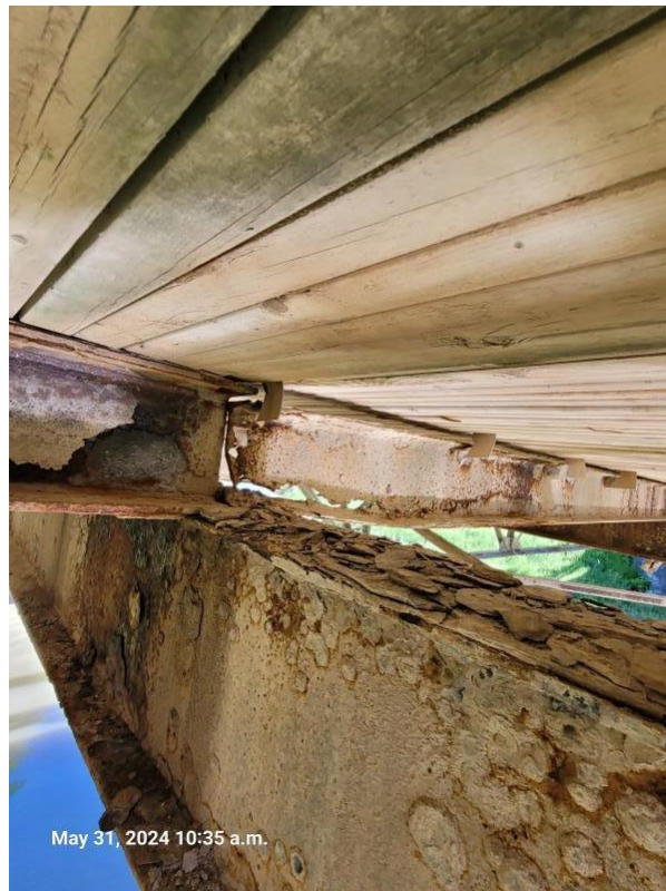
8-Crossbeam and Corroded Stringer
