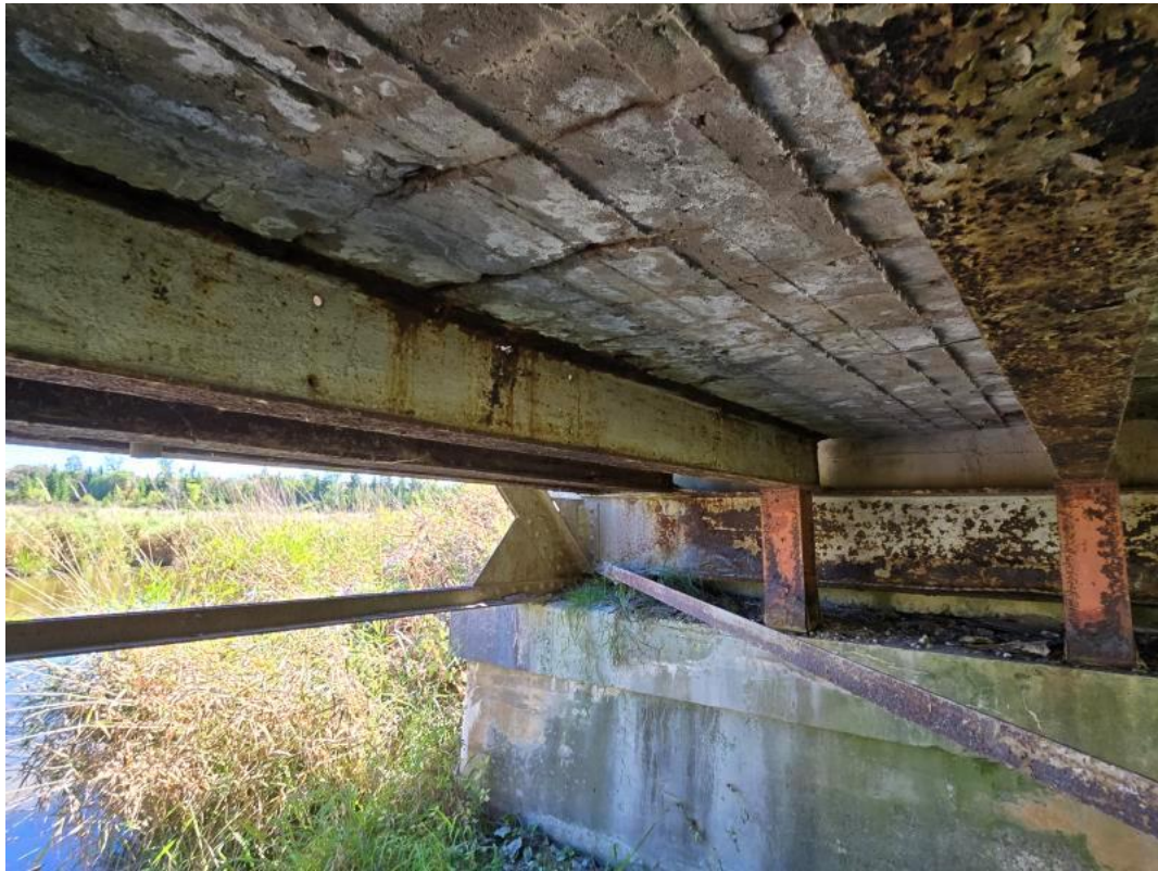
South Bay Corroded Perforated Web
