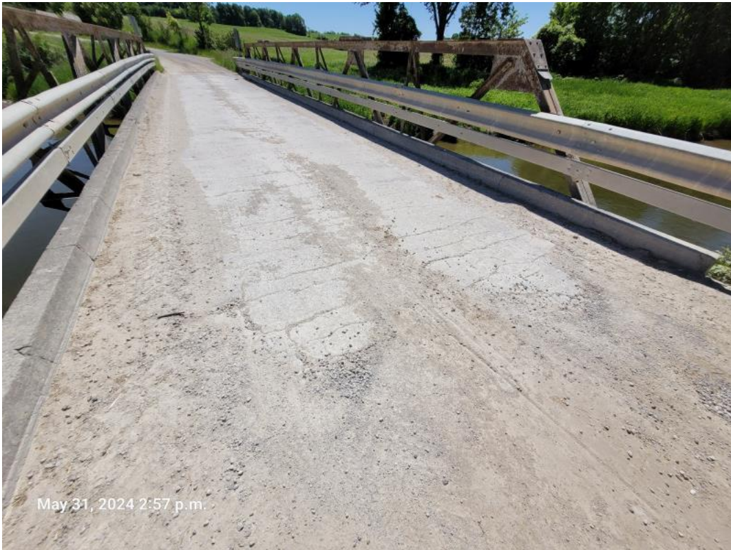
Deck Top Cracks
