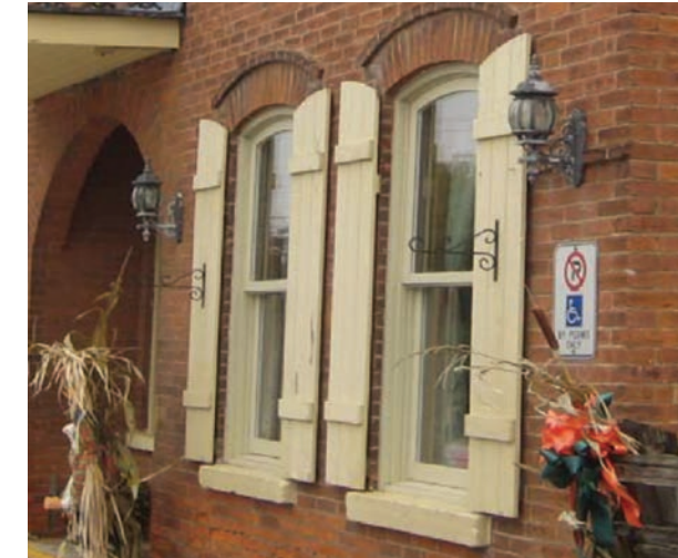
Arched board & batten shutters fit the window shape.
